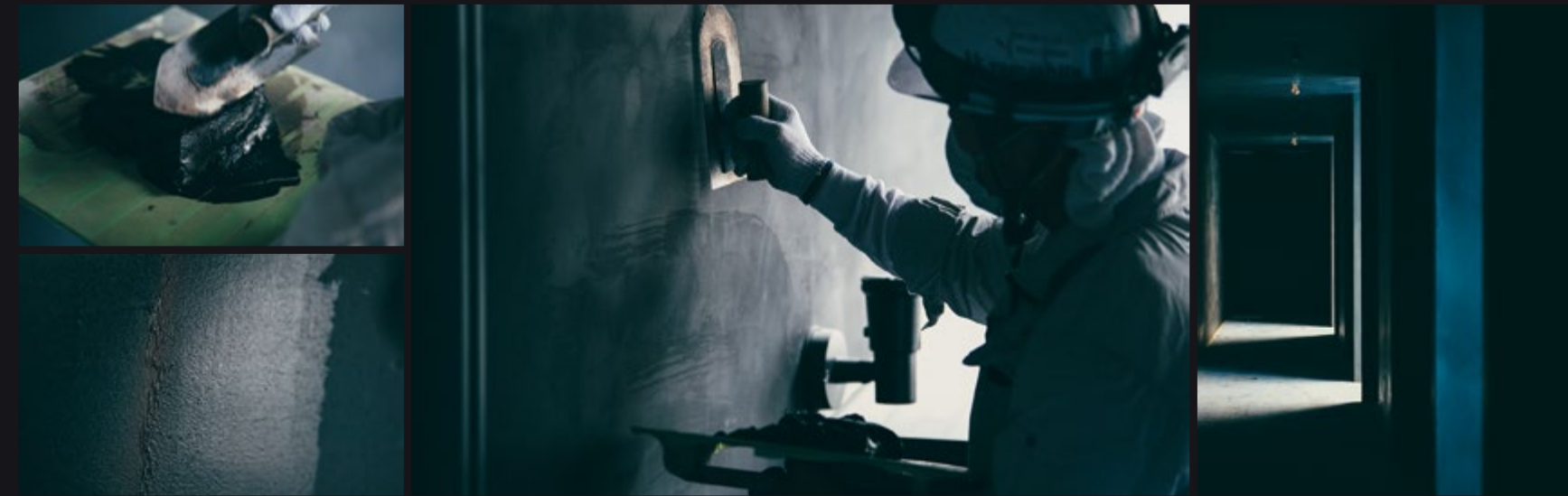
墨漆喰…漆喰に墨を混ぜて塗りあげる、伝統的な左官工法のひとつ。左官塗の中でも難易度が高く、職人の技術が問われる仕上げである。 Black ink plaster: one of the traditional plaster-making processes is to mix black Japanese ink with plaster and apply it. This is an extremely difficult finish which requires great ability from the artisan.
