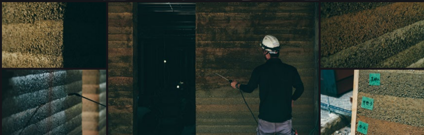
版築…杉板の型枠を組み、赤土、中塗り土、真砂土といった三種類の土を10cmの厚さ毎に突き固めることによってつくられる。版築を突き固めた後に型枠を外し、仕上げとして表面の吸水性を抑えるため樹脂を吹き付ける。 Rammed earth: it is built by assembling a mould from Japanese Cedar board and ramming down 3 different types of earth, red, medium coarse and fine sand earth every 10 cm. After being compacted down in the formwork, the mould is removed and resin is sprayed to limit the water absorbency of the surface.
