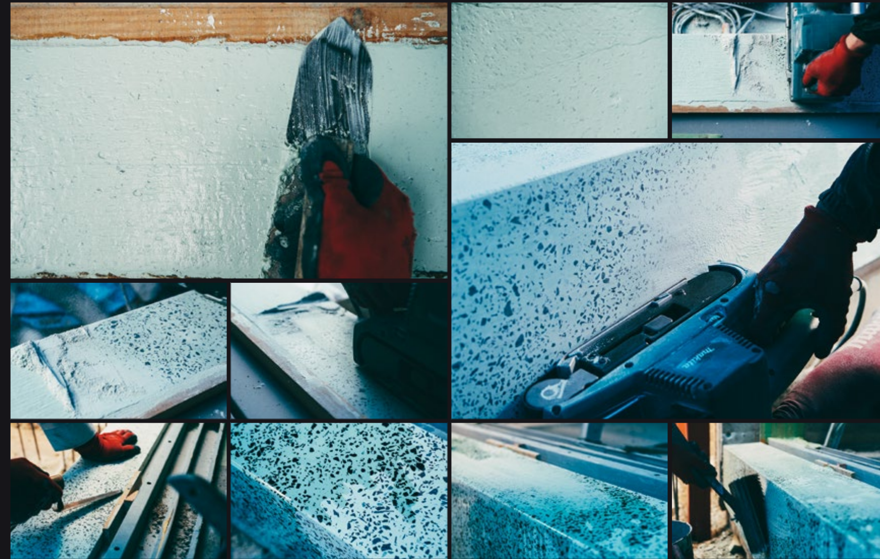
研ぎ出し…白セメントと緑色をした大理石の一種である蛇紋石を混ぜてコテで塗った後、磨きあげる左官仕上げ。光沢のある研ぎ出しの質感と版築の荒々しい表情が対比をなしている。 Polished terrazzo: white cement and the green marble “serpentine” variety are mixed together, applied to the surface with a spatula and then are polished with a grinding machine. The feeling of the glossy polished concrete is juxtaposed to the rough expression of the rammed earth.
