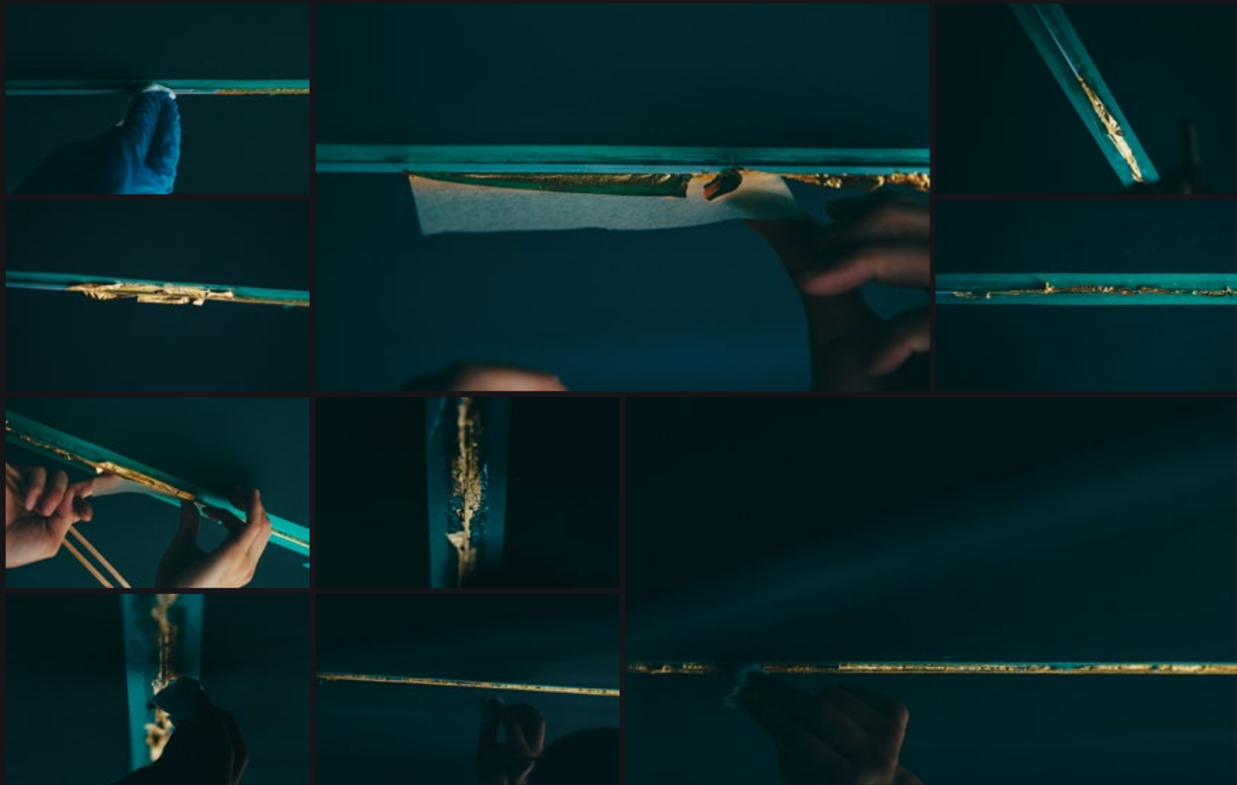
金箔貼り…躯体に溶接された3mm幅のステンレス・フラットバーに、注意深く養生を行いながら、吹けば飛ぶほど繊細な金箔を手で貼り付けていく。 Gold leaf fixing: a gold leaf so thin that it could be blown away is very carefully transferred by hand to the 3 mm wide stainless-steel flat bar welded to the framework.
